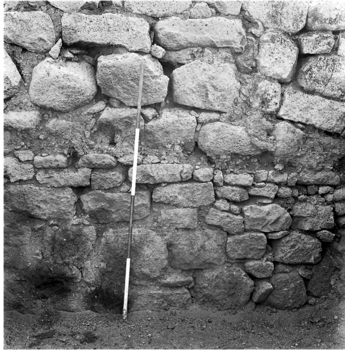
1. Detail of the southeastern wall of room E5 in Building E, view from North-West.
