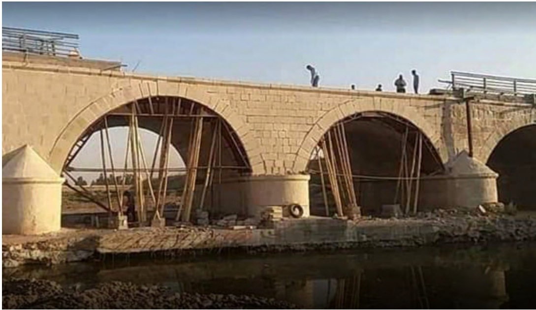
1. Centre of lower Khosr bridge under repair. View from south, c. 2019. Image by Aamir Fadel, 2020, Google Maps.
