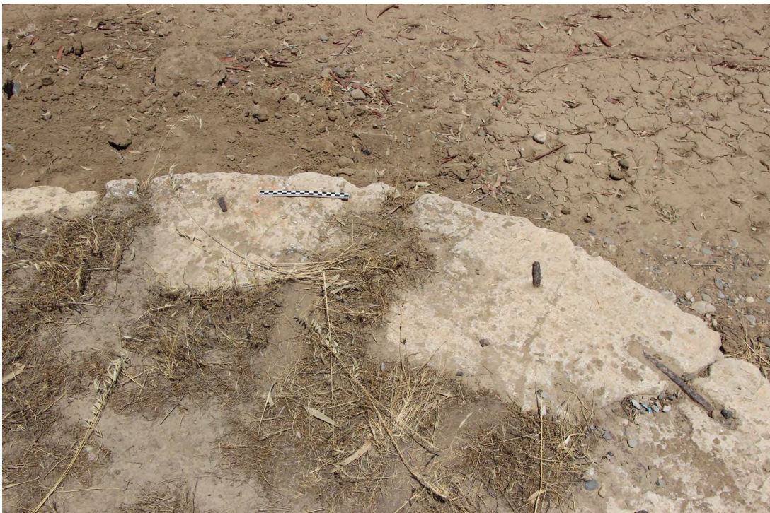
2. Iron plug protruding from a hole in a sixth course ashlar of Pier 3.
