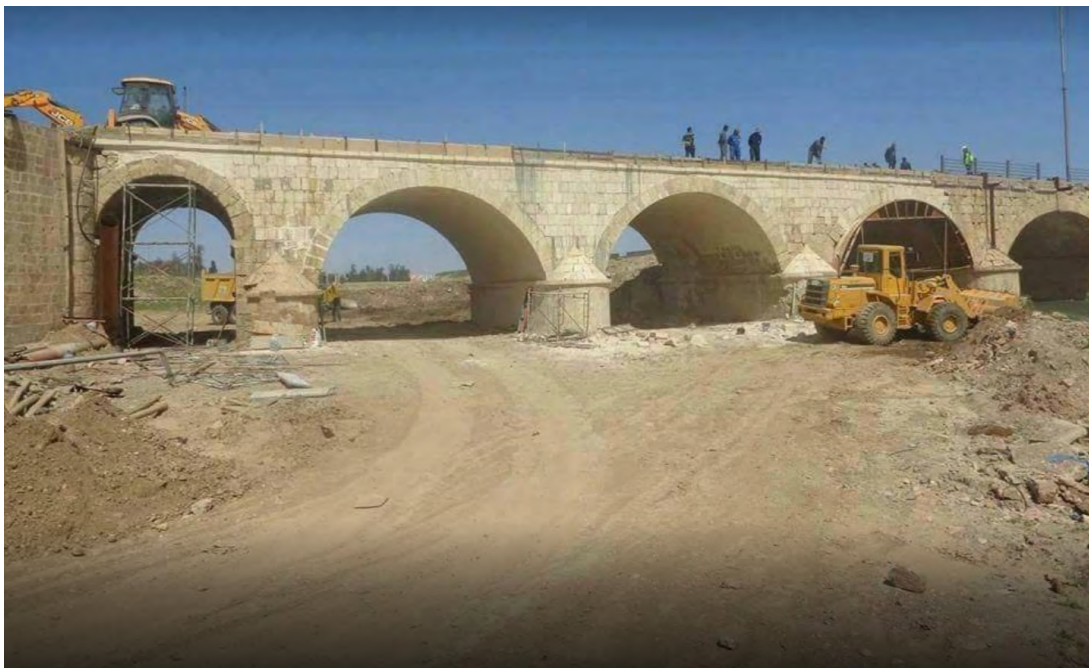
2. East end of lower Khosr bridge under repair. View from south, c. 2019. Image by Adnan Adnane, 2020, Google Maps.
